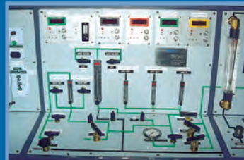
Job 473 Year 1997 Panel Hyperbaric Treatment Chamber - Taiwan Hospital
