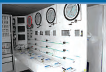
Job 700 Year 2004 Sat System Control Panels, Electrical Panels & Container
