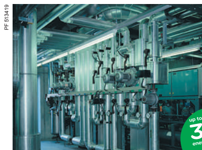
ATV12 controlling a pumping station
