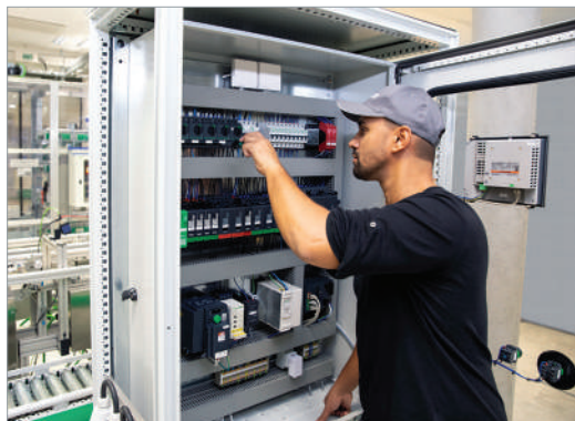
General machine control
